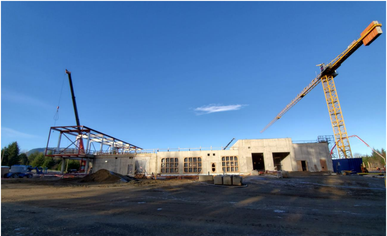
Water Treatment Plant east side – from left to right: Lobby, Flash Mixing, Chemical Tank Area, Sludge Dewatering, Electrical Room
