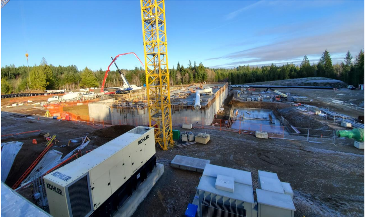
Foreground: Water Treatment Plant Generator and Unit Substation Background: Clearwell with Backwash Equalization Tank foundation starting on right
