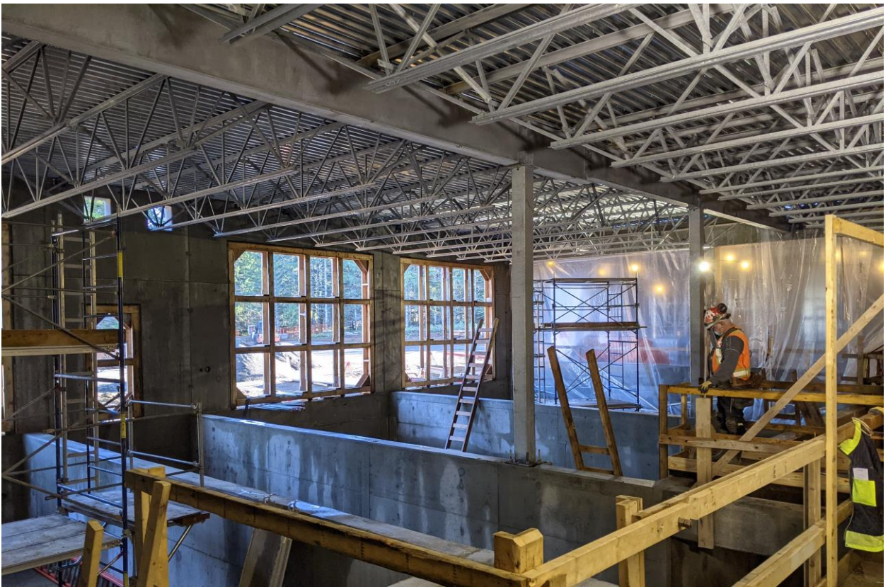
Water Treatment Plant Chemical Tank Area – ready for tanks and overhead doors
