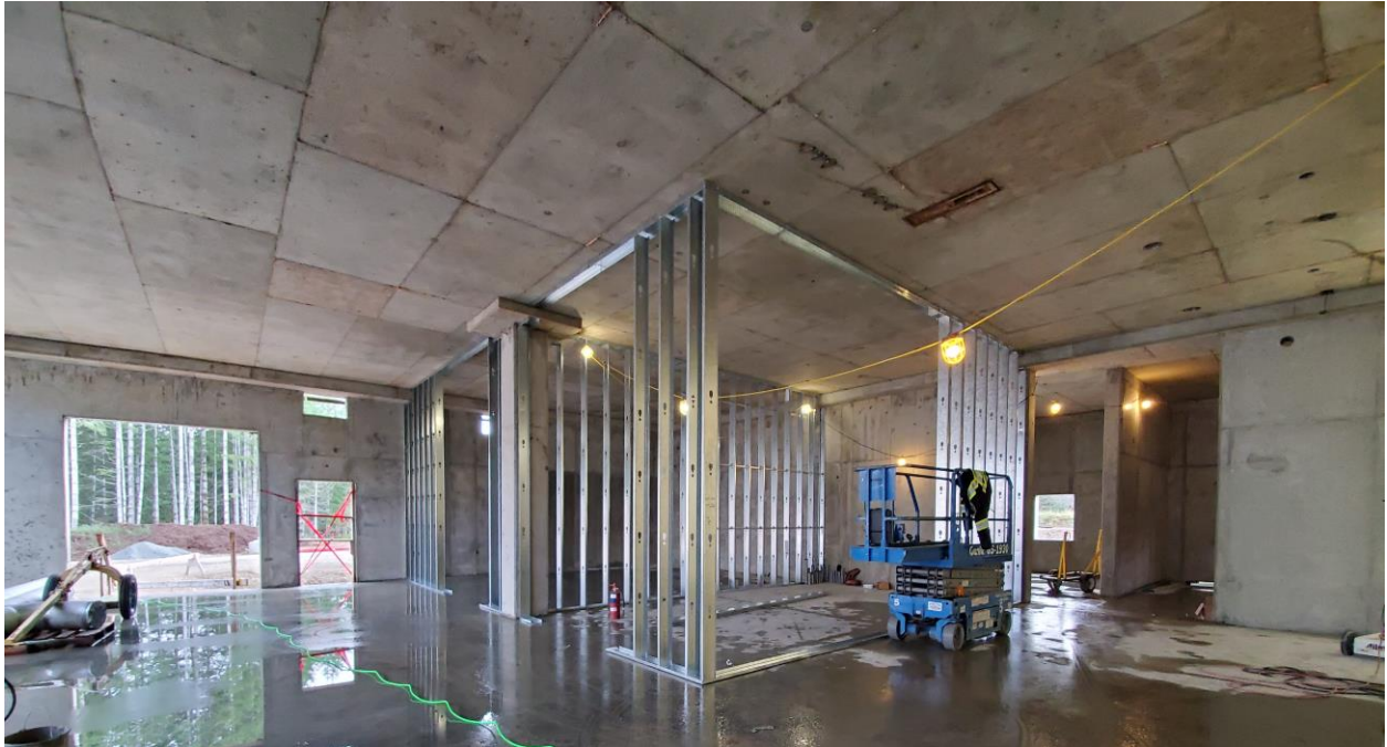
Inside Water Treatment Plant – Building Mechanical room walls being installed in Flash Mixing area
