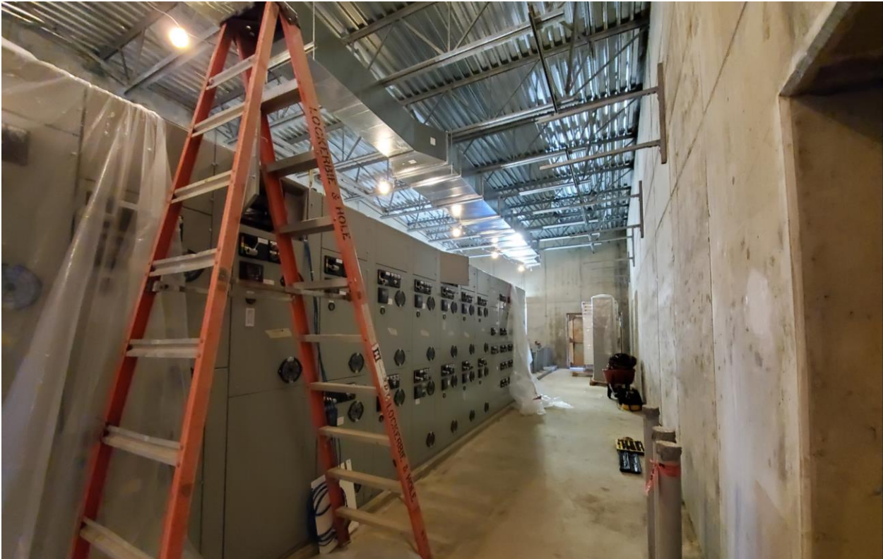
Water Treatment Plant Electrical Room
