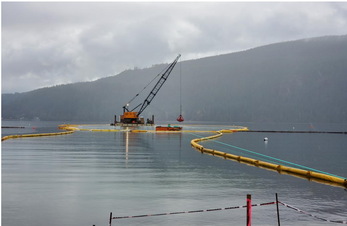
Dredging in Comox Lake – preparing lake bed for submerged portion of Marine Pipeline
