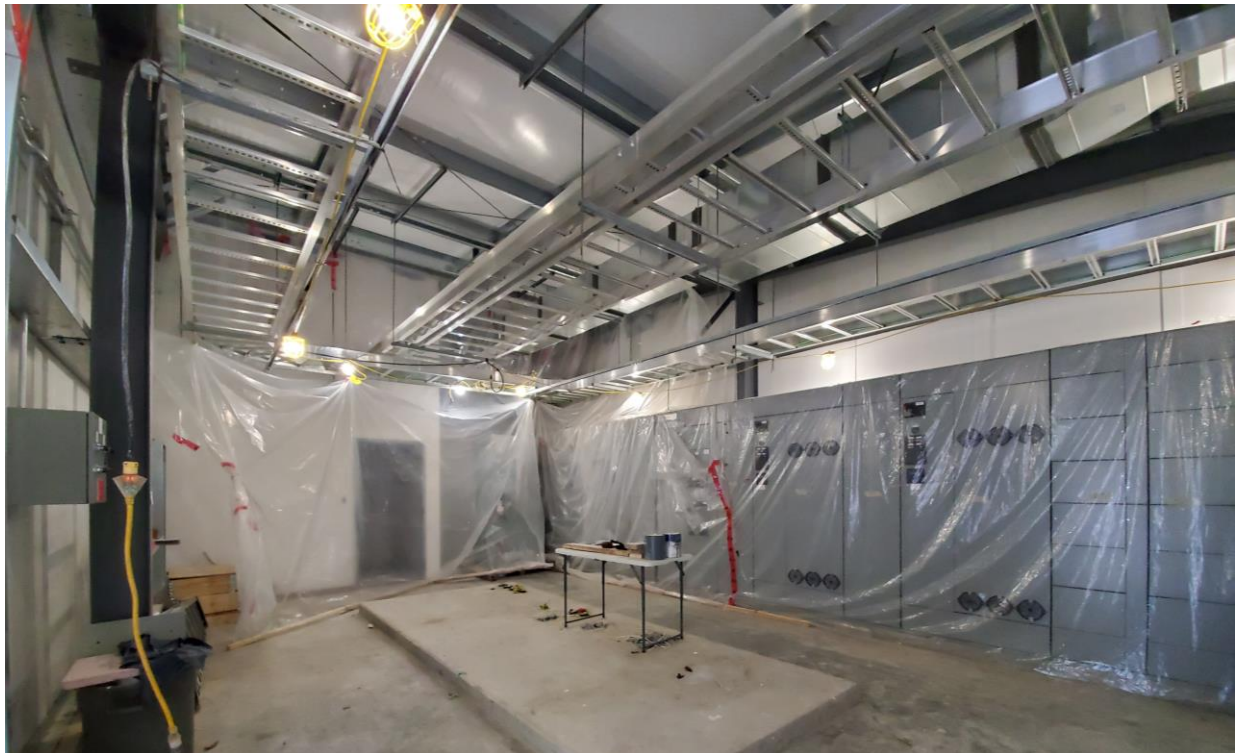
Raw Water Pump Station Electrical Building – MCC Cabinets installed ready to be energized
