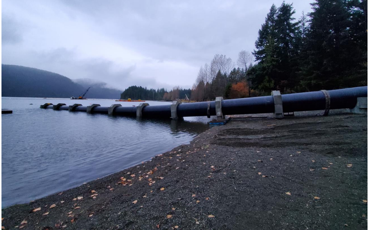
HDPE portion of Marine Pipeline – welded and ready move and to sink into place
